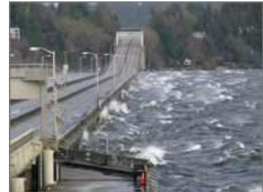
Waves batter pontoons of SR 520 bridge Pontoon Project
